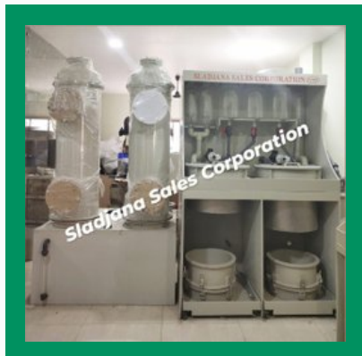
Gold Refining Plant
